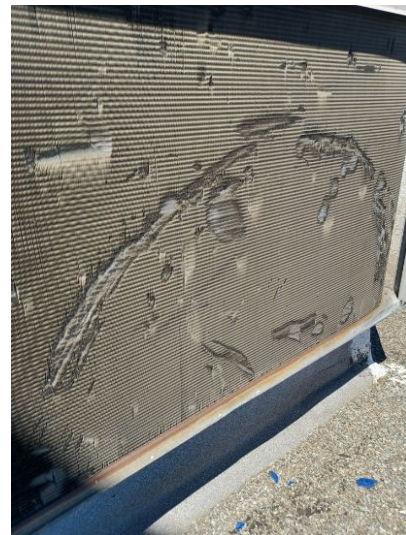
Damaged fins noted to units
