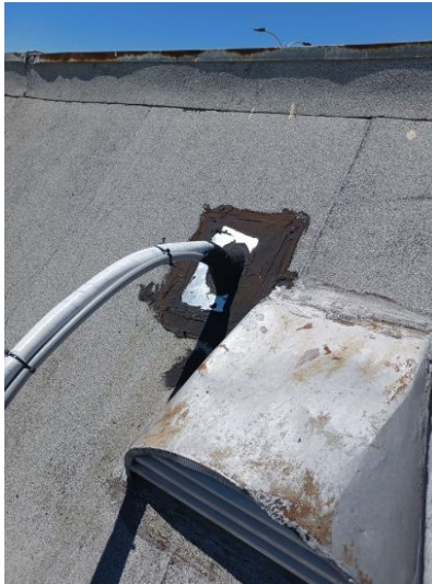
The flashing around the rooftop heating/cooling system is only mastic around the edges which is not a reliable long term seal. This will be a higher maintenance item.
