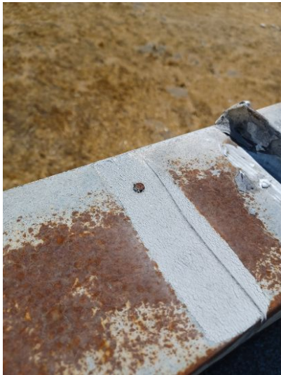
The parapet wall flashing is in poor condition.
